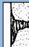
Mortar smeared over the face of the stones produces a half rendered effect
