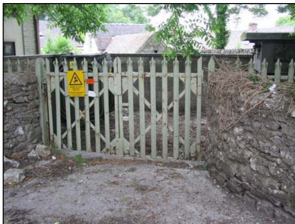
P129 Electricity sub-station by Memorial Hall
