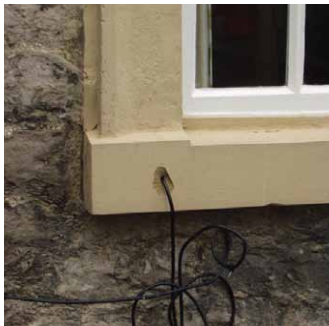
This picture shows the effect of a poorly sited cable and the damage done to an historic window, by insensitive drilling
