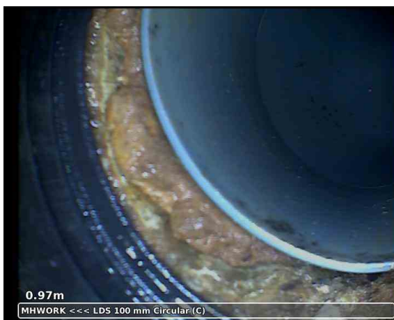
20240211-234549-snap0002.jpg, 00:00:23, 0.97 m Survey abandoned, Rest Bend - Disabled WC and Ladies
