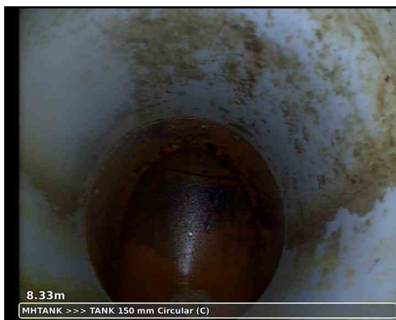
20240212-002705-snap0002.jpg, 00:00:55, 8.33 m Finish node, other special chamber, reference: TANK, Septic Tank
