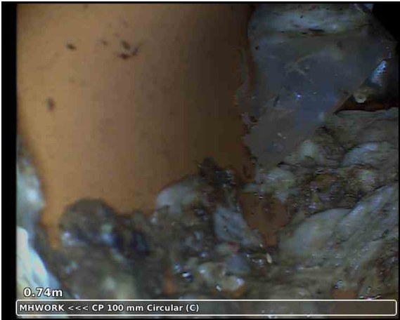
20240211-234448-snap0001.jpg, 00:00:13, 0.74 m Survey abandoned, Capped Off
